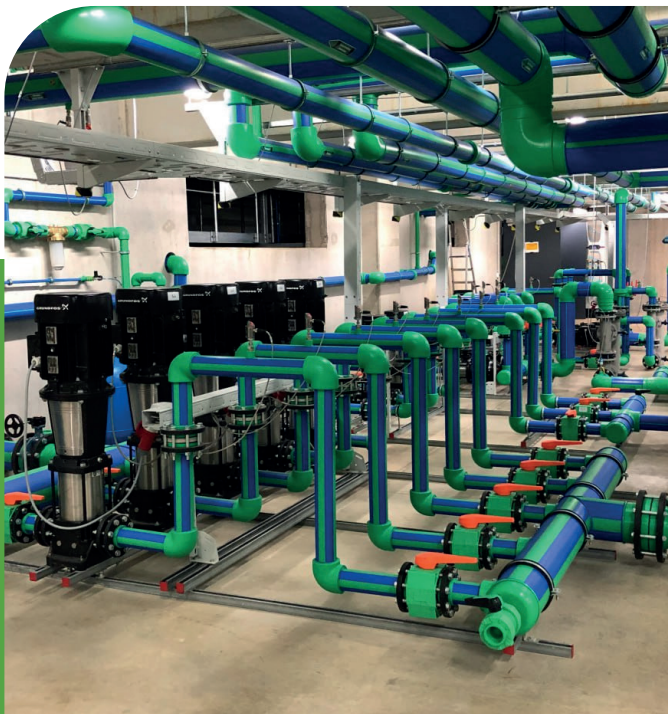
Transfer Pumps (Cold Water System)
