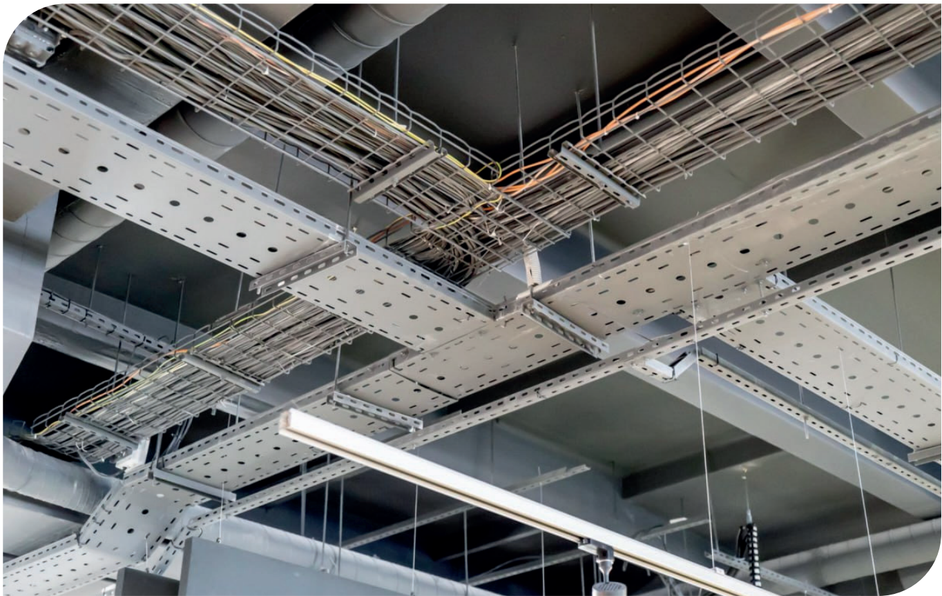
Electrical Cable Tray
