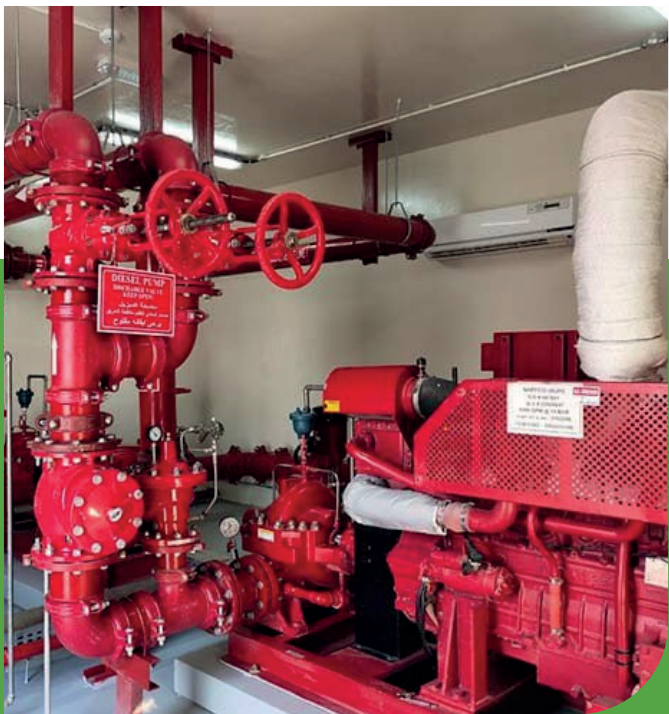
Fire Fighting System
