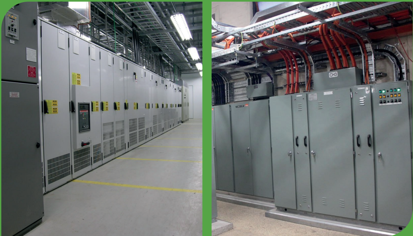
Main Distribution Board
