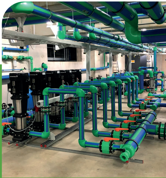
Transfer Pumps (Cold Water System)
