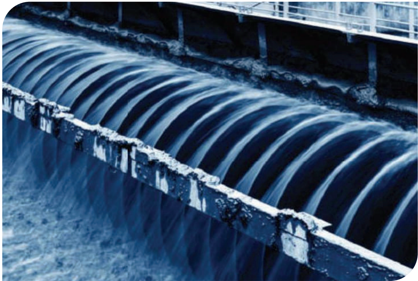
Water Treatment System
