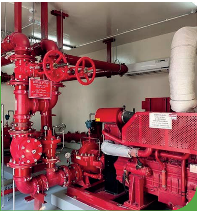
Fire Fighting System
