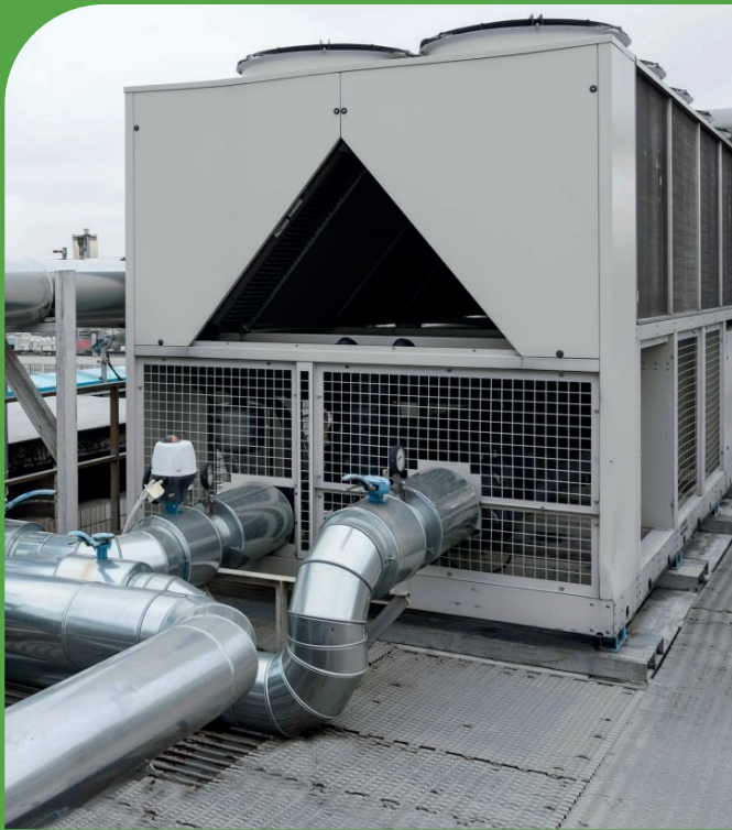
Air Cooled Chiller System
