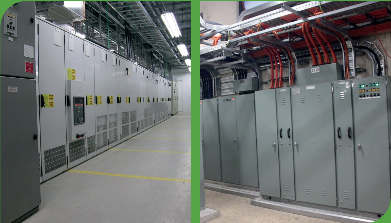
Main Distribution Board
