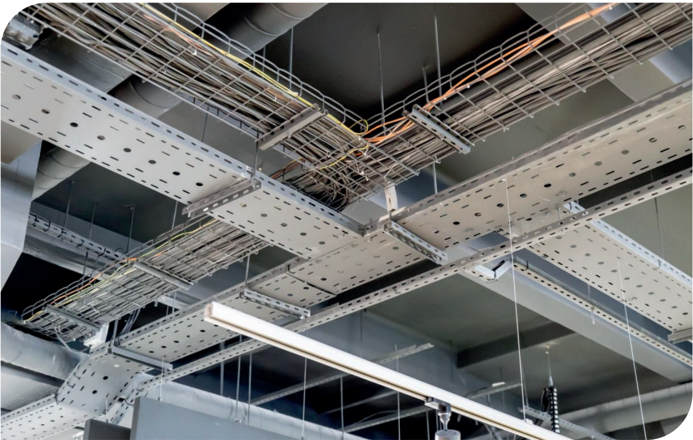
Electrical Cable Tray
